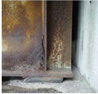
Photo 1: Corrosion of transverse stiffener.
