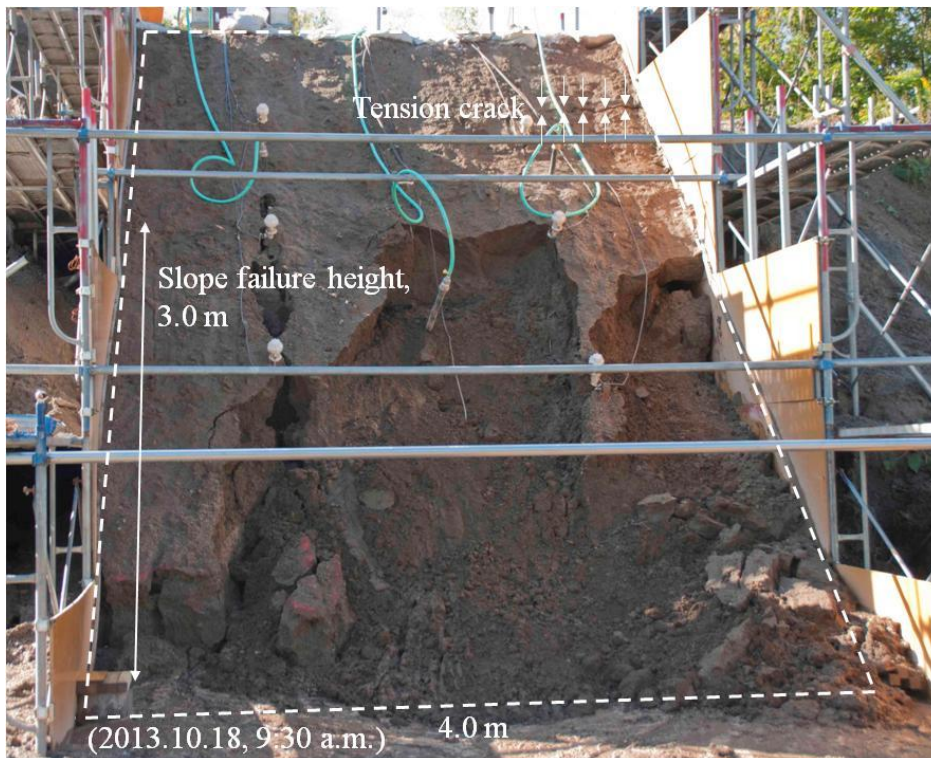
(a) Slope failure of FE-2012 immediately after the occurrence on 2013.10.18
