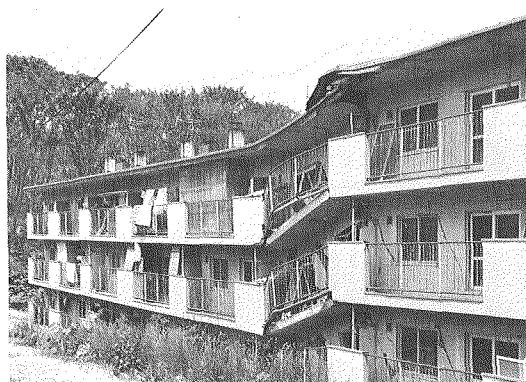
Photo. 4. Damaged building situated on a fissure formed by the 1910 eruption, at Point D in Fig. 4 (b). (photo. Sept. 1978)
