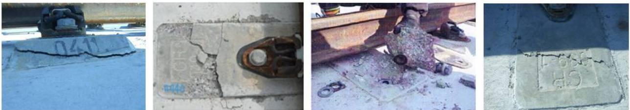
Figure 1: Cracks developed in the railway sleeper
