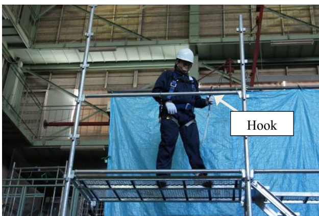
Figure 11: The worker who tried setting the guardrail between the supports.
