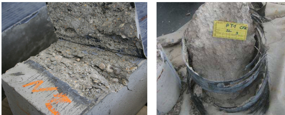
Figure 1: Destroyed concrete beam and column after failure of CFRP material.
