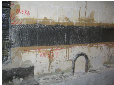
Figure 19. Sliding along the mortar bed
