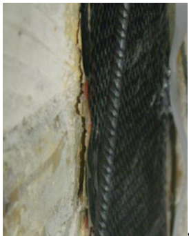
Figure 18. Delamination at the top of the column
