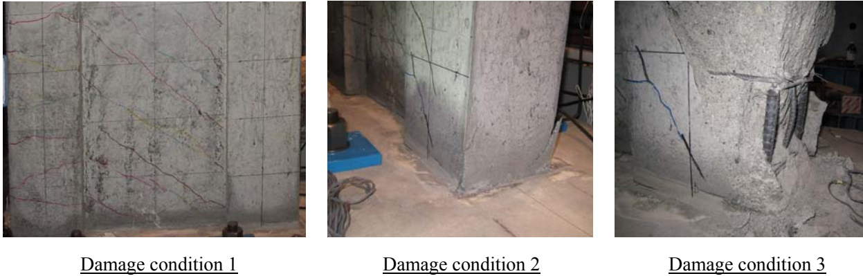
Photo 2: Damage condition (Specimen No. 1)
