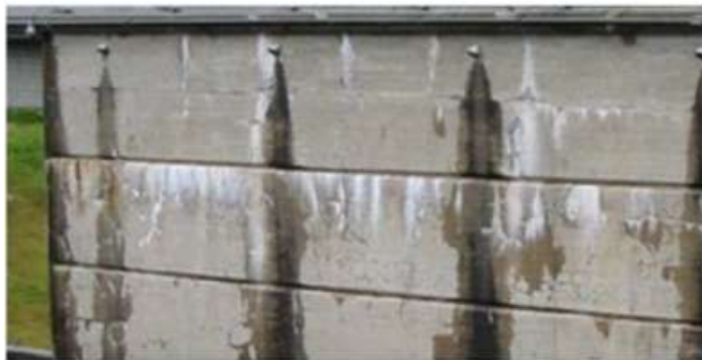
Fig. 1.2 Cracks with an opaque white coating on surface of dam [1]
