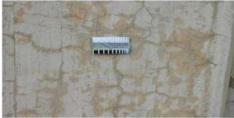
Fig. 1.1 Map cracking pattern on the surface of dam [1]
