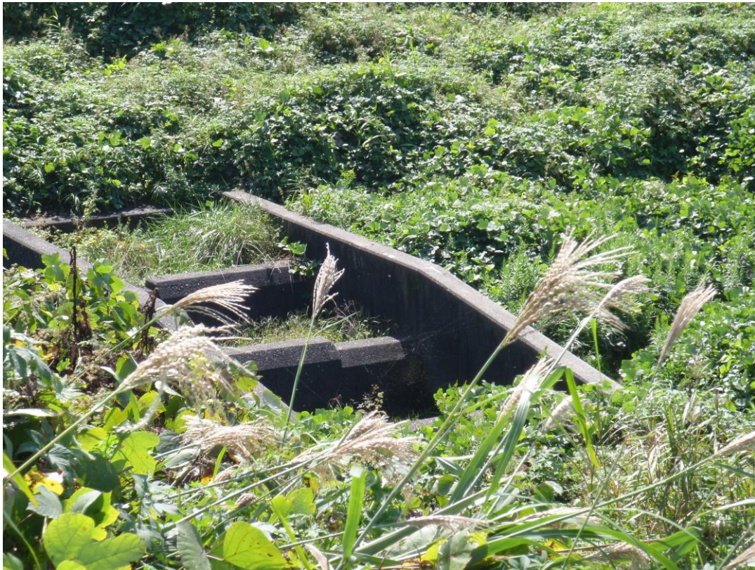
Fig.6-5. Fish ladder, which lose function by sand drift.
