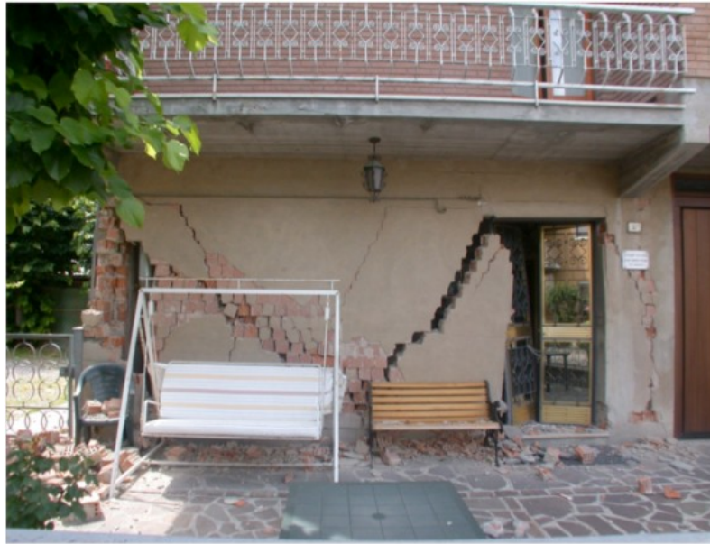
Fig. 5.7. Typical diagonal tension failure in a squatting wall during Emiliana Earthquake in Italy, 2012 (EAI 2012)
