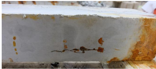
(c) Corrosion crack after finish second accelerated corrosion
