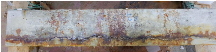
(c) After finish corrosion for the second time
