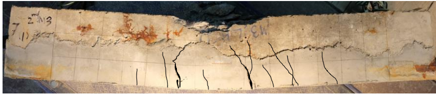
(b) The beam repaired with method 3
