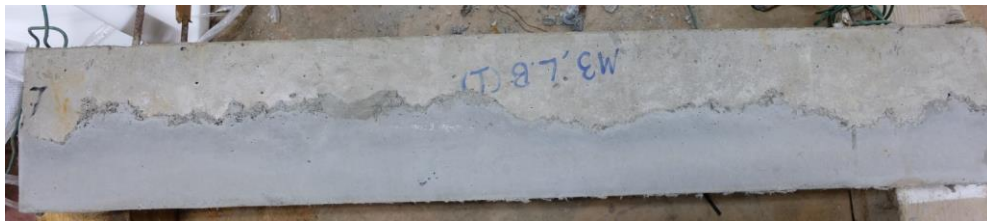
(a) After finish corrosion for the first time and then the beams were repaired with method 3
