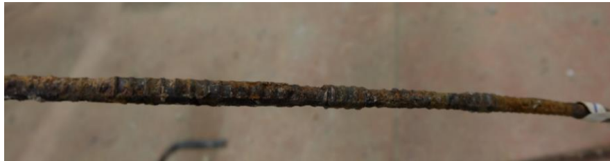
(a) Steel bar corrosion for the beams in group 1
