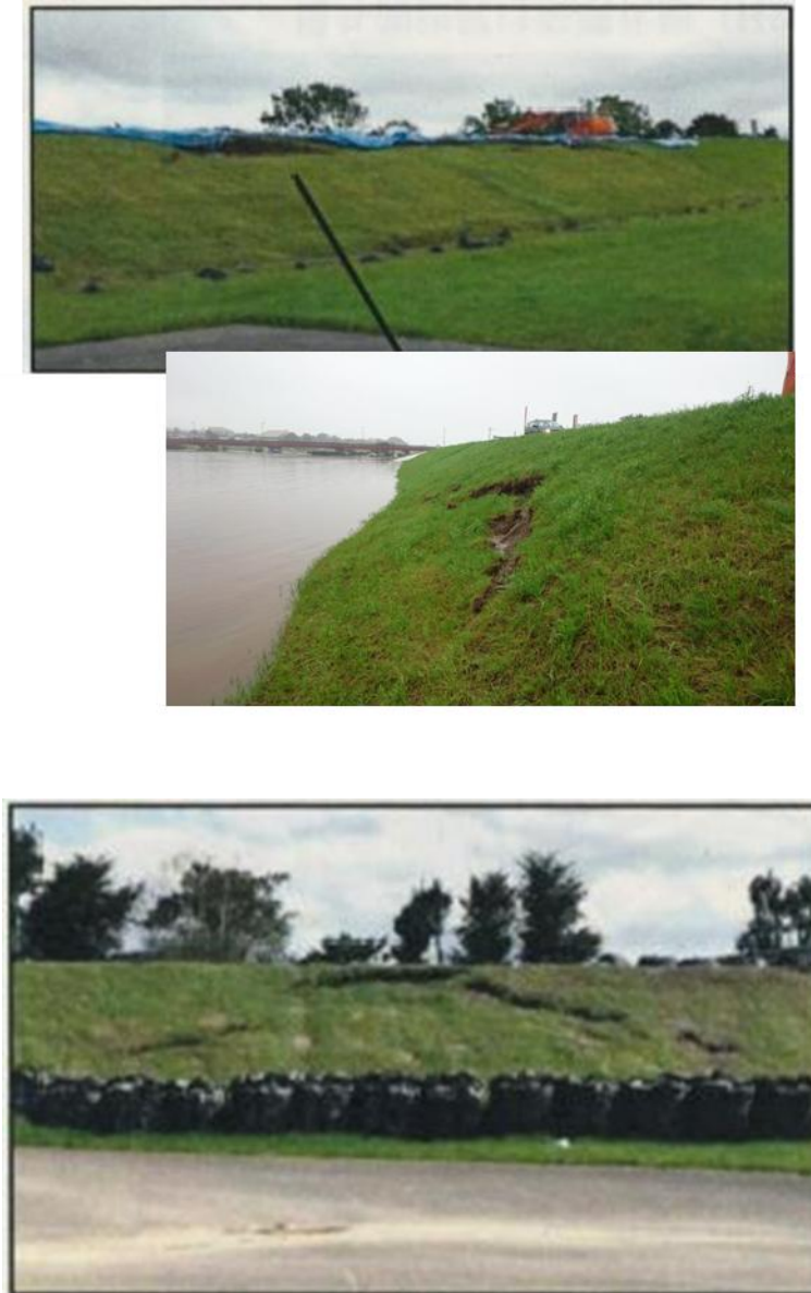
Figure 3.1. Photographs showing shallow slope failure in Kushi River dyke due to heavy rainfall in August 2016 (Source: Final investigation report by the Japanese Geotechnical Society Hokkaido Branch)
