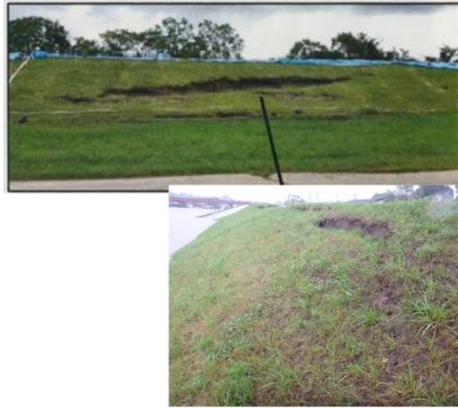
Figure 2.2. Photographs showing shallow slope failure in Kushiro River dyke due to heavy rainfall in August 2016 (Source: Final investigation report Japanese Geotechnical Society Hokkaido Branch)
