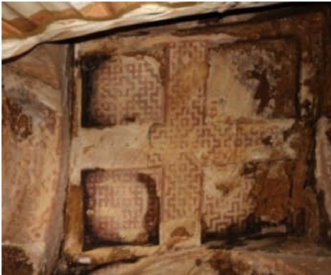
Fig 4. 26. A deteriorating ceiling decoration
