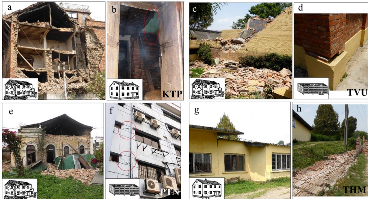
Figure 3. 17 Damaged structures around the seismic stations.
