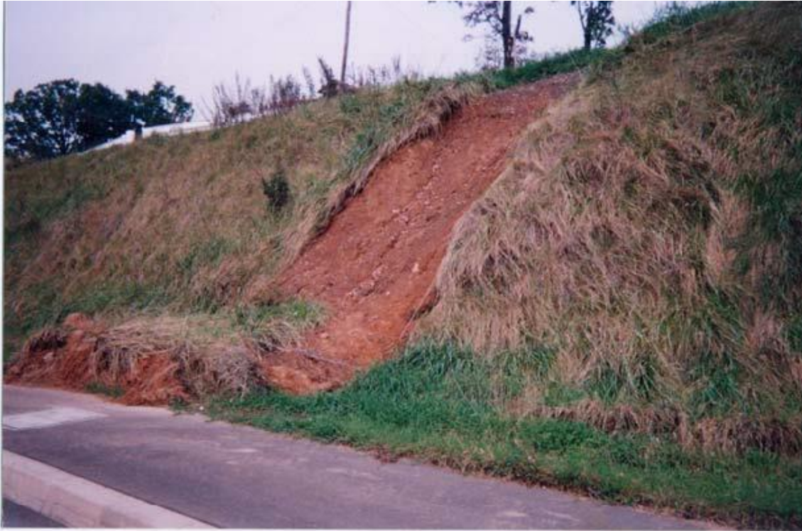
Figure 1.4 Surface collapse of slope due to thaw settlement (After. Ueno et al., 2010)
