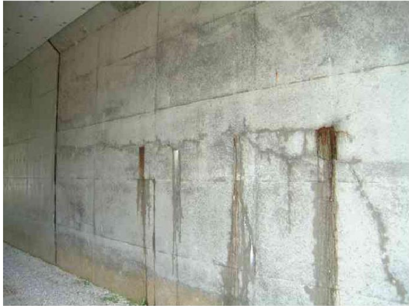
Figure 1.2 Horizontal cracking in the sidewall of culvert (After. Hayashi et al., 2006)
