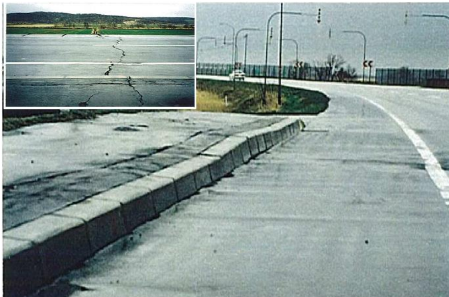
Figure 1.1 Frost-induced pavement roughness and cracking (After. Hayashi et al., 2006)
