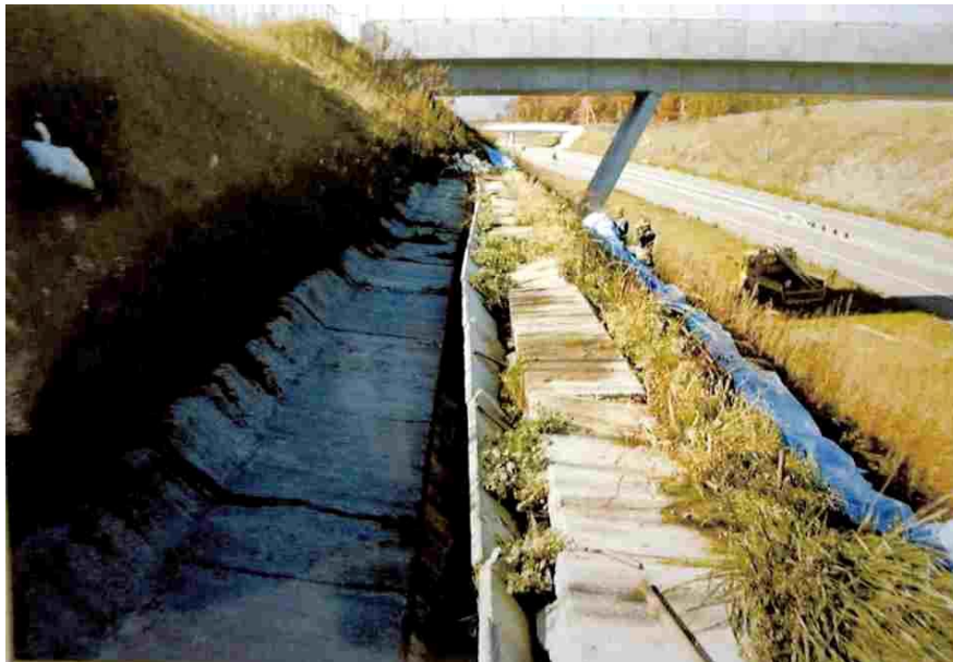
Figure 1.3 Frost heave damage of the small stage drainage (After. Tozuka et al., 2006)
