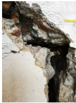
(a) Steel fracture in tension
