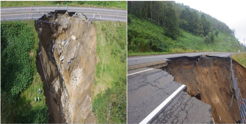
Figure 2.5 Slope failure at Route No. 38, Hikachi Pass, Hokkaido, Japan on 31 August, 2016.
