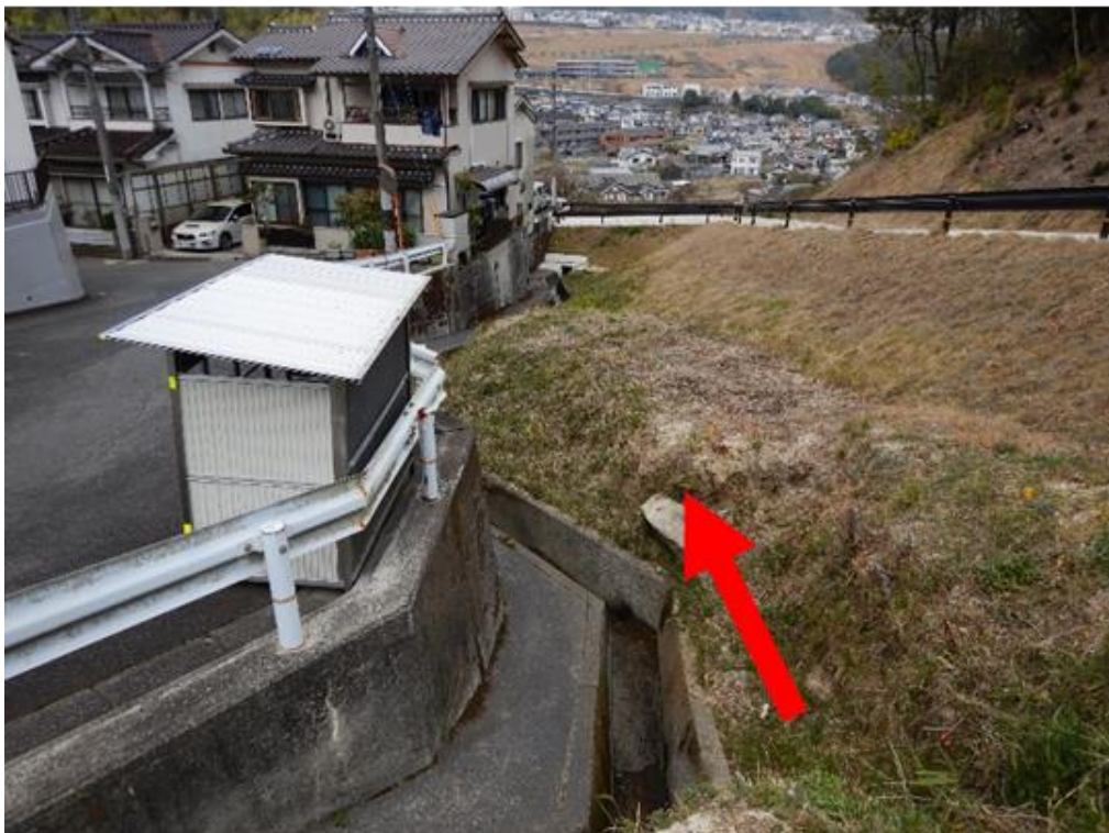
Fig. 1-7. Insufficient scale of drainage (Hiroshima, Japan)
