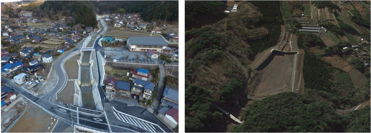
Fig. 1-5. Countermeasures against the SSF (Left: Channel works, Right: Sediment basin)
