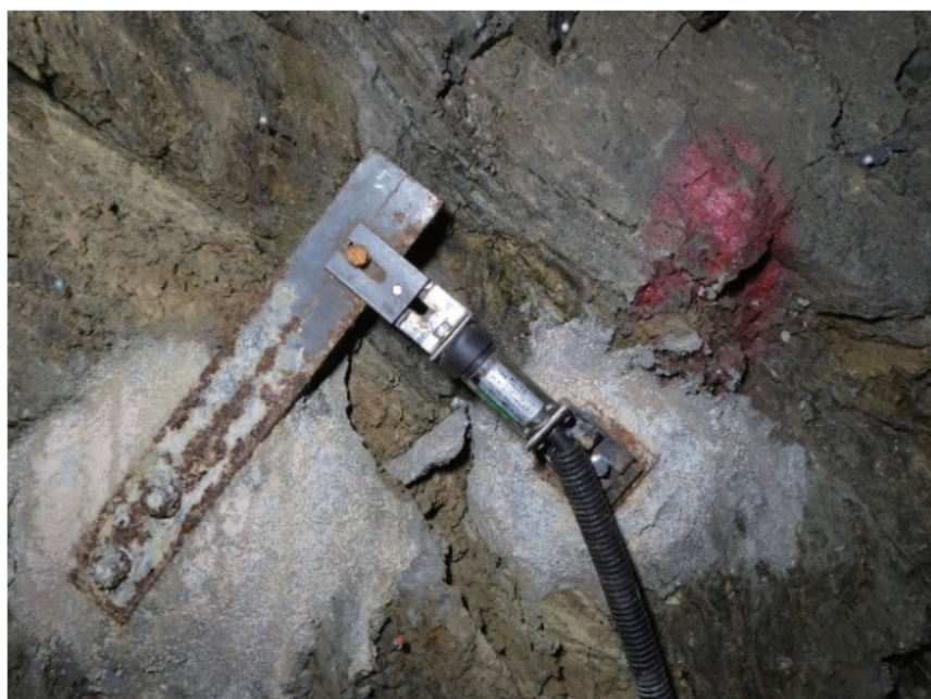
図 2 - 2 3 Close-up of No.5 fracture (with crack gage).
