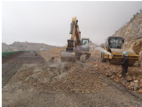
(c) The area of cement reinforcing on the front side of rock piling.
