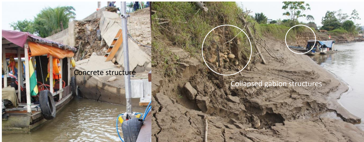
Figure 4.8: Bank protection measures in the Ichilo River. Left: Concrete structure, right: gabions.
