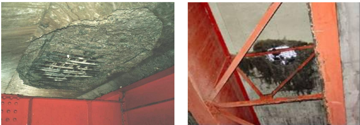
Figure 1.1 Punching shear failure of bridge RC slabs
