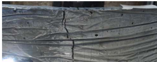
(c) Crack localization under the bottom of UHPFRC layer at final failure
