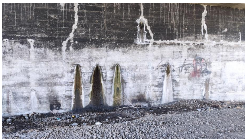
Figure 5.6 Water leakage of bridge 1704
