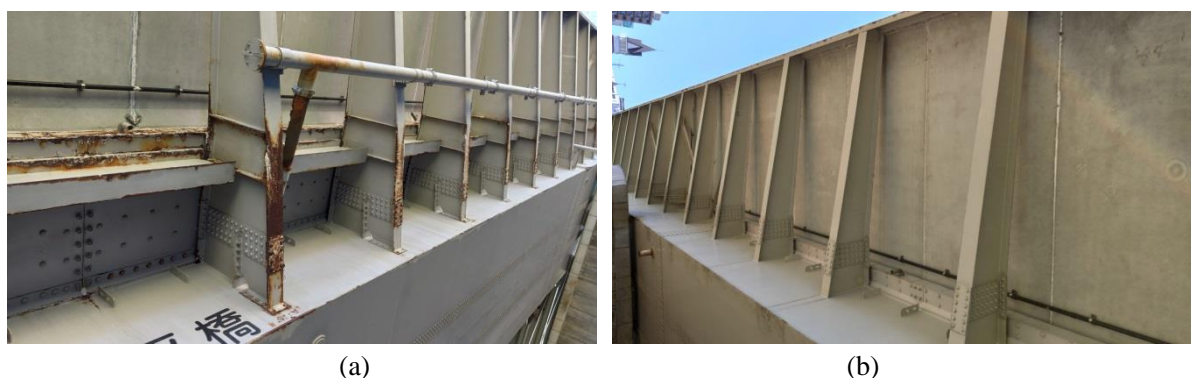
Figure 5.7 Corrosion of the bracket on the (a) north side and (b) south side.
