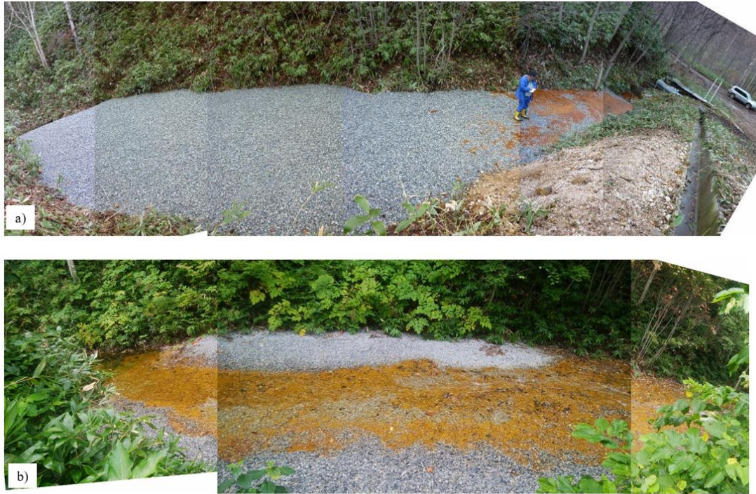
Fig. IV-1. The figure of the open limestone channel at the Shojin wastewater discharge, a). the OLC just after the construction, the photo was taken on 2017/11/14, b) the OLC after 296 days after the construction (2018/09/05).
