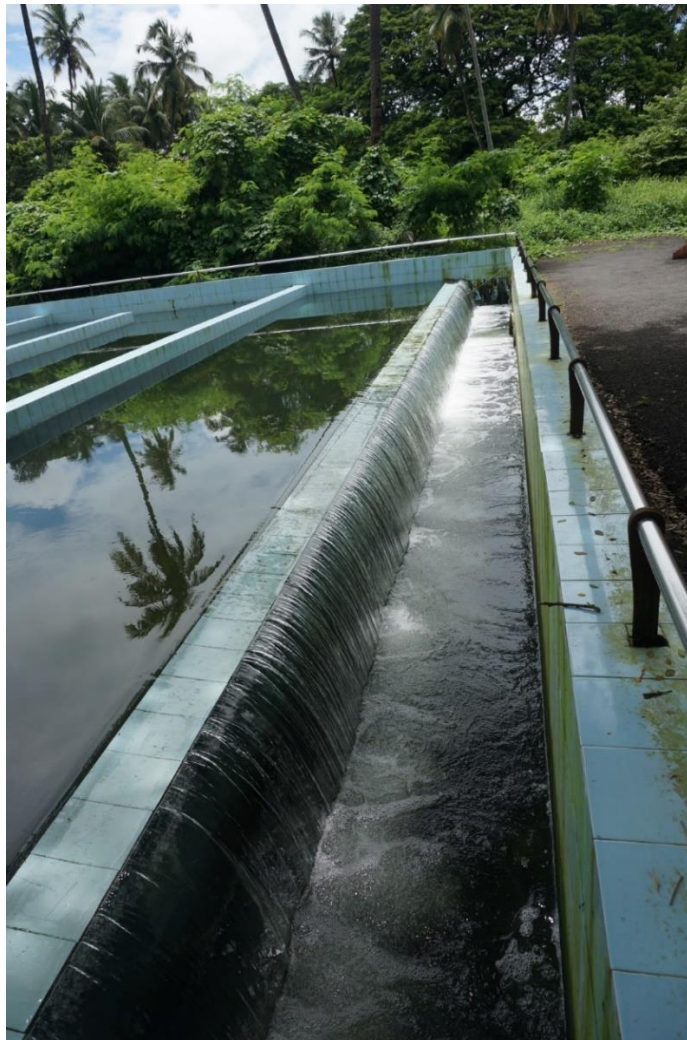
Fig A9. Decantation tank in Tonca Sewage treatment plant. Treated wastewater of ecologically safe quality being discharged. Photo taken during October 2020
