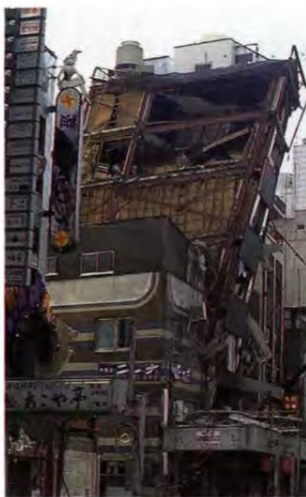
Figure 2.2: Heavily damaged seven-story braced frame building (source: NIST [8]).
