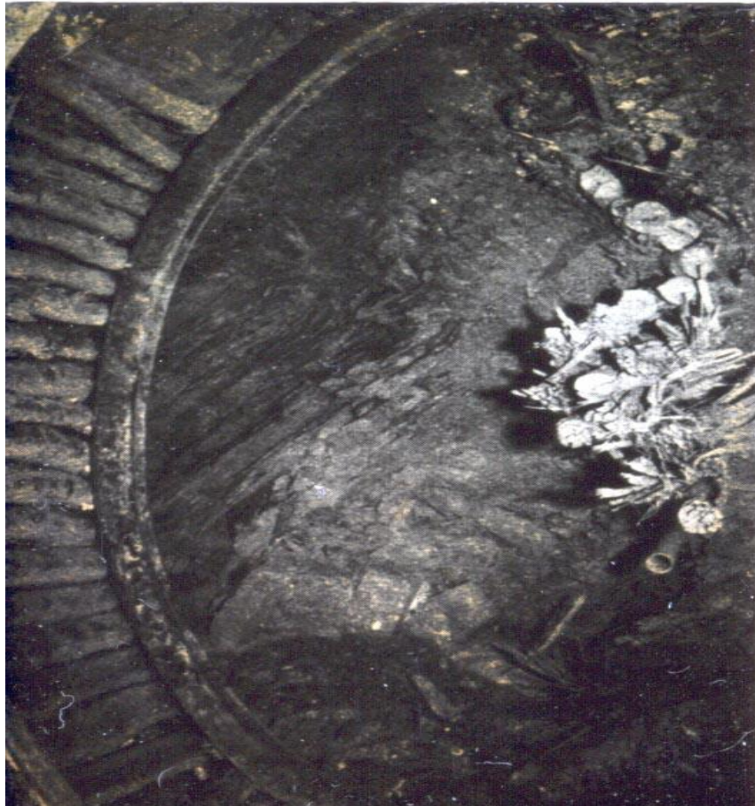
Fig. 1.1 Intensely damaged steel set supported drives at Kolar Gold Fields. [Photograph from Fairhurst (1988) and Caw (1956)].
