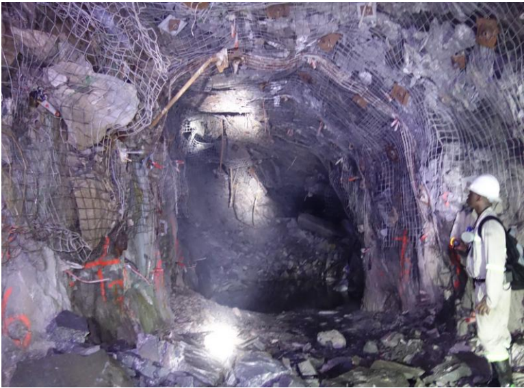
Fig. 2.8 Rockburst site for M2.8 (date taken: 15th March 2018).
