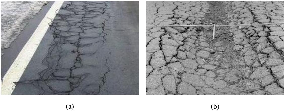
Figure 1-1 Types of pavement damage in in seasonally cold region ((a)Fatigue cracks; (b) Rutting).
