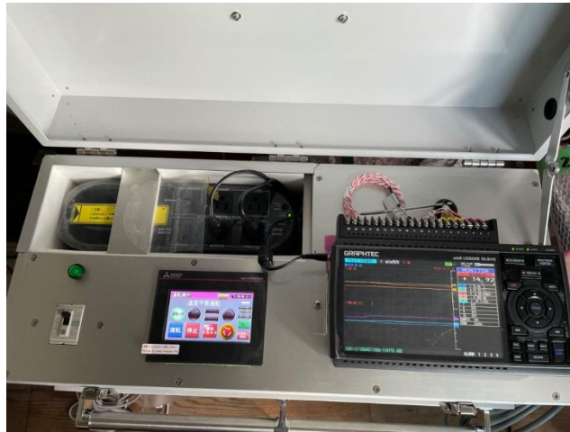
Fig. 3.14 Devices used for TRT test.
