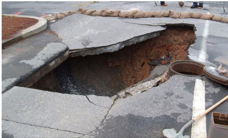
(d) Collapse due to rainwater leaking through pavement and carrying soil into a ruptured sewer pipe. Source: https://handwiki.org/wiki/Earth:Sinkhole
