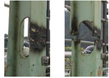
Half-Cut Full-Cut Figure 2. Damaged members
