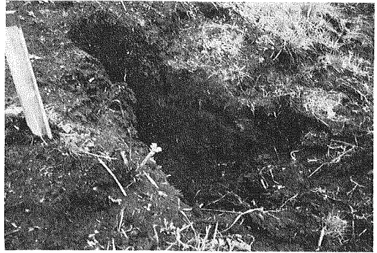
Photo. 7.2. Large crack on slope
