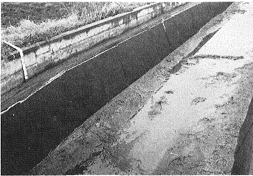
Photo. 2・1. Concrete lining channel made height increasing for settlement (Hokkai north main channel)
