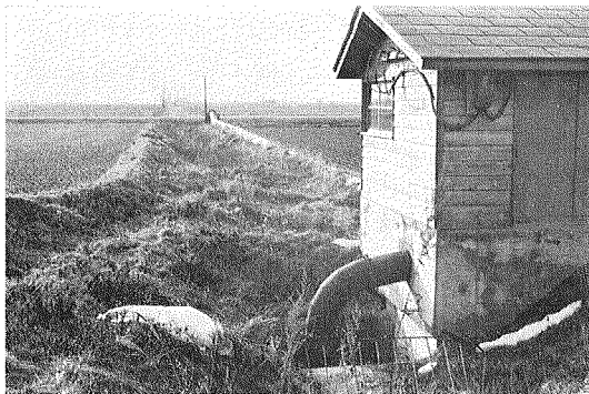
Photo. 2・2. Pump-station for assistant supply (Kawamukai main channel)
