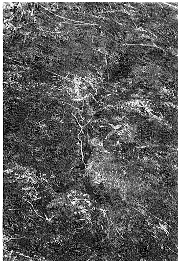
Photo. 7.1. Crack on slope
