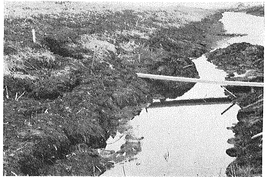
Photo. 7.3. Collapsed slope caused by crack
