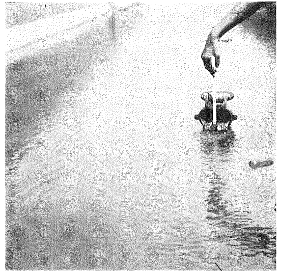
Photo. 6.2. Vertical weep hole located in bottom wall is connected to underdrain
