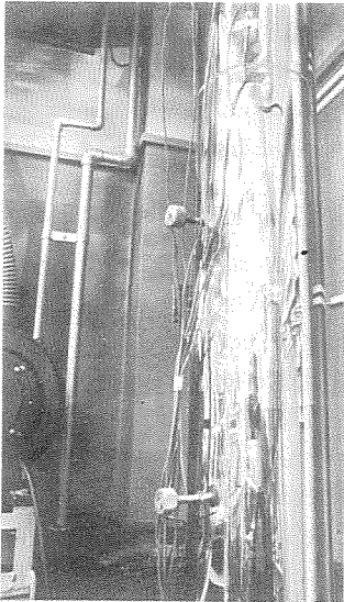
Fig. 4. Heat exchanger. (Surface is covered with insulator)
