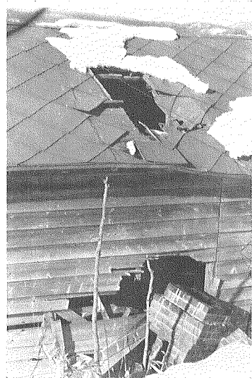
5 煙筒の倒壊 Collapse of a chimney
