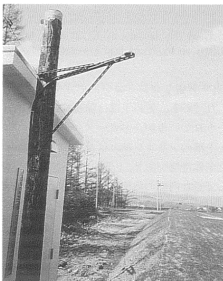
Photo. 2(b). GPS antenna put on the end of steel arm fixed to the wooden pole. Strainmeter electronics, data logger, and sensors of atmospheric pressure, ambient sub system temperature, dialup-communication system, and PC are set inside the hut being 30 m distant from the well(Photo. 2(a)).
