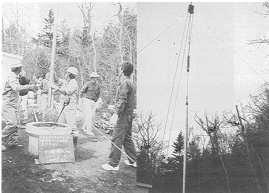
Photo. 3. Installation of the sensors at KUT(left). Strainmeter and 3-comp seismometers lifted up by crane and lowered to the bottom of the well at KUT(right).
