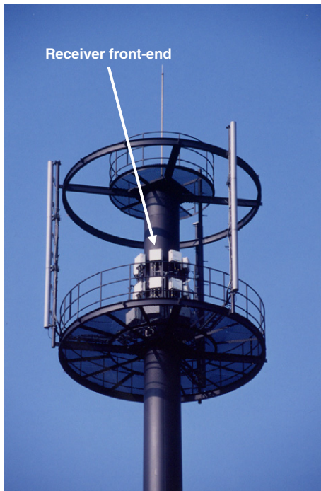
Figure 2. An example of a tower-mounted receiver front-end.
