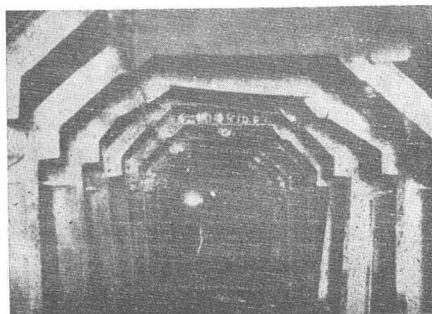
Pl. II'. The construction deformed by "earth-pressure."
