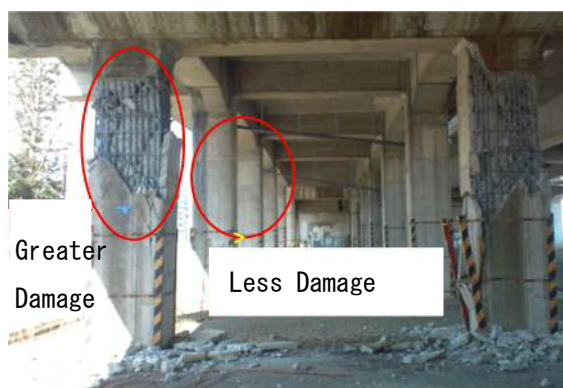
Fig.1 Damage of Shinkansen ramen viaduct (Minami Nagamachi in Tohoku Sendai) after the Great East Japan Earthquake
