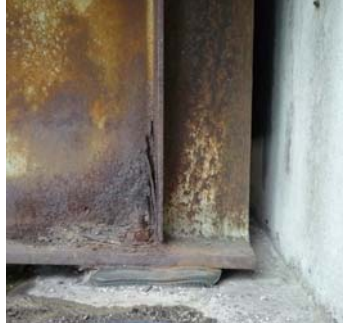
Photo 1: Corrosion of transverse stiffener.
