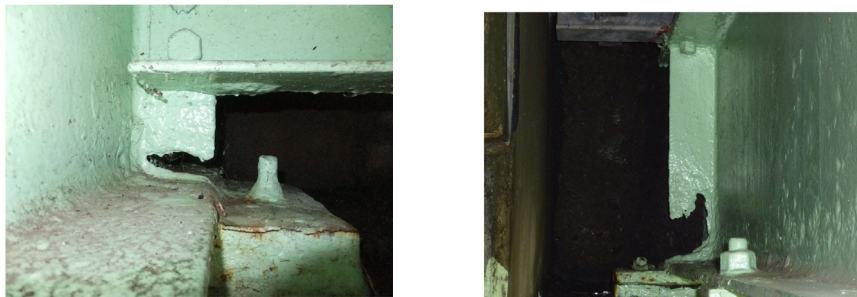
Figure 1: Examples of corroded girder ends
