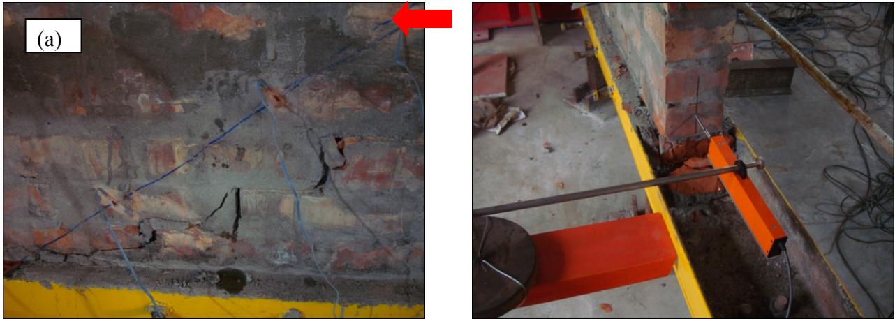
Figure 7: a) Crack opening displacement and b) crushing at wall toe for RW2
