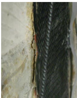
Figure 18. Delamination at the top of the coulum
