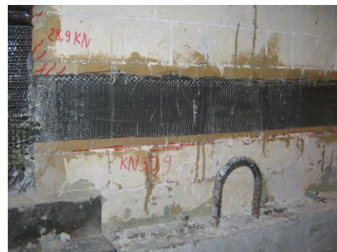
Figure 19. Sliding along the mortar bed
