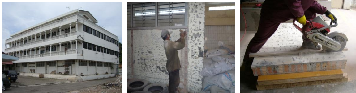
Photo 2: Damaged building and preparing specimens.
