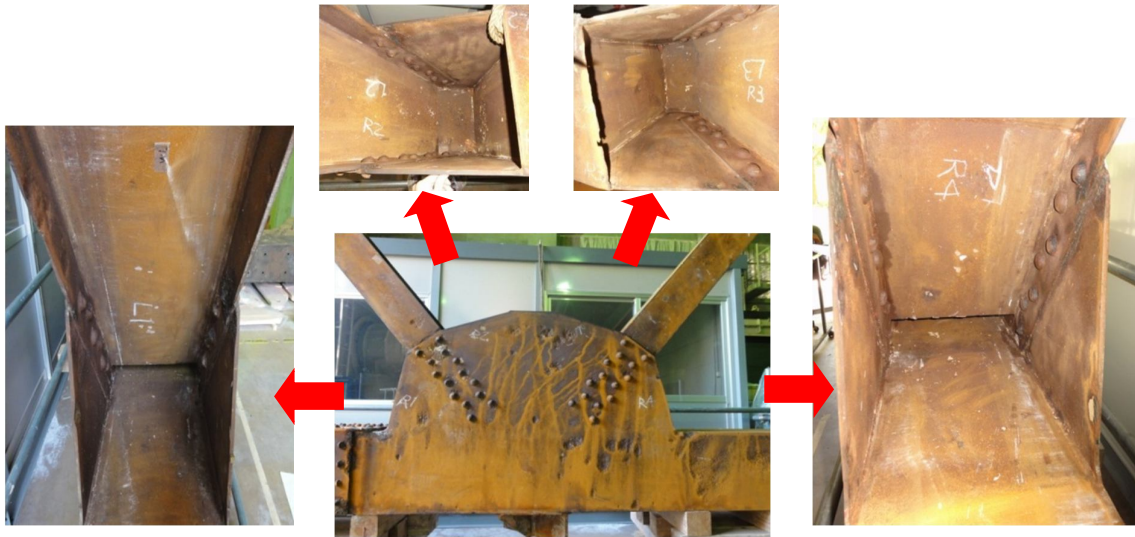
Photo 4: Corrosion condition of the inner surface of narrow section
