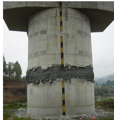
Fig. 1.4 Bridge pier damage in earthquake
