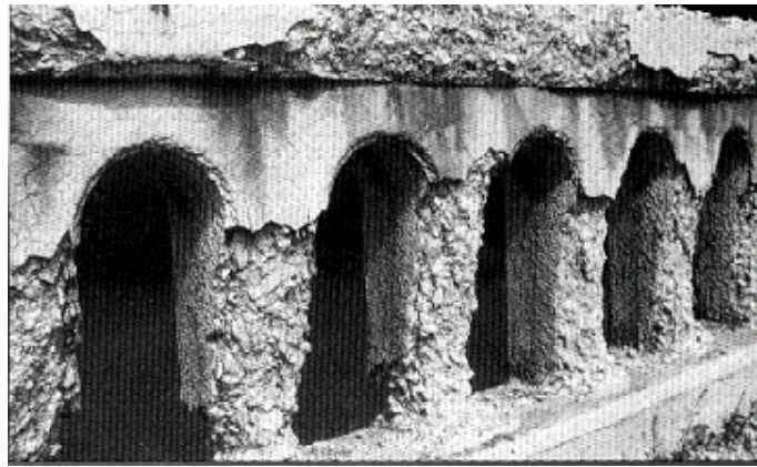
Fig. 1.1 Frost damage of the concrete structures
