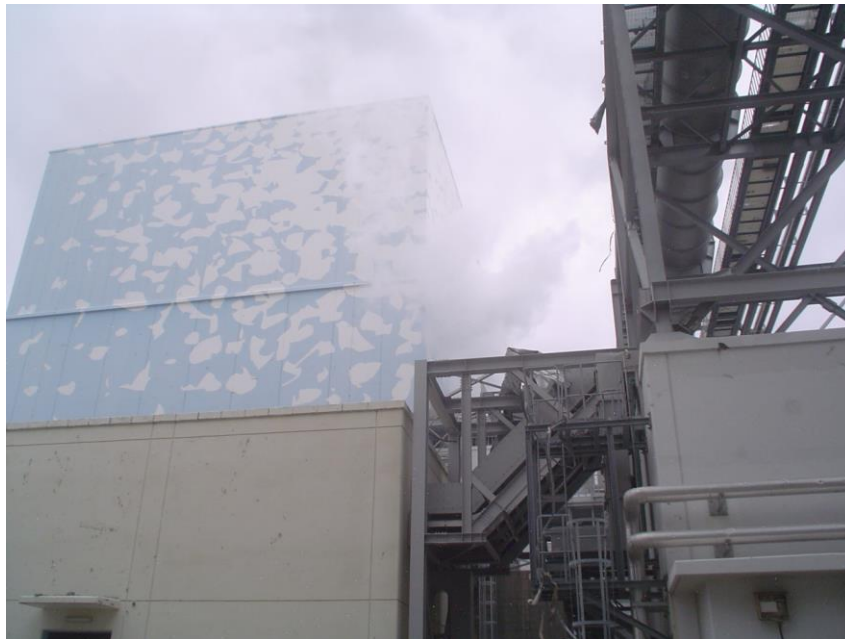
Fig. 2-3 Steam coming out of a blow-out panel opening at the Fukushima Dai-ichi Unit 2 Reactor Building on March 15, 2011. The photo was taken at 8:59 AM on March 15, 2011.
