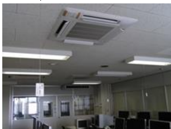
Fig. 6.11 Indoor units of conventional system (back) and developed system (front) at Shizuoka (Hitachi-Johnson Controls Air Conditioning, Inc.)
