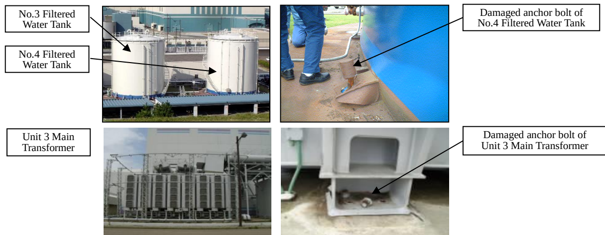
Fig. 4-6 Anchor bolts fracturing of Filtered Water Tank and transformer
