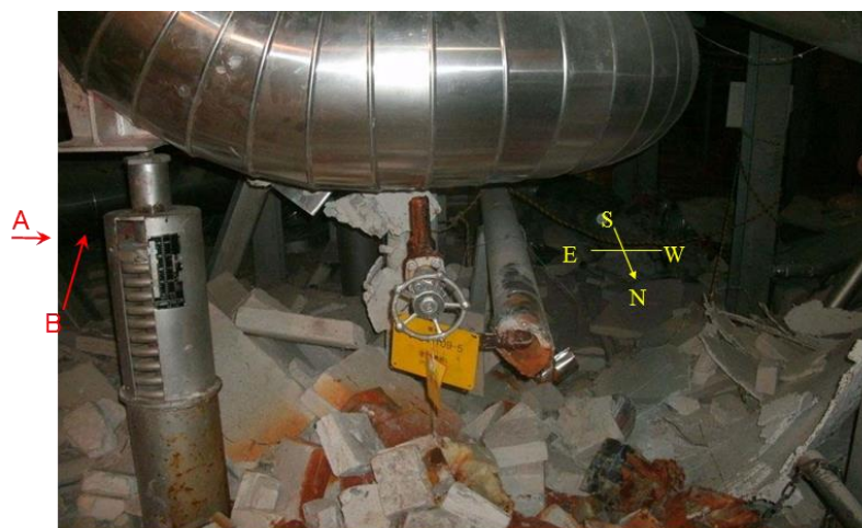
Fig.3-6 Photo of Moisture Separator after the earthquake
